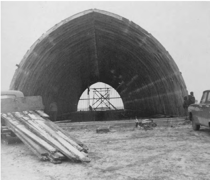
Lowe Farm Curling Rink under construction in 1959. It was entirely a volunteer effort.
